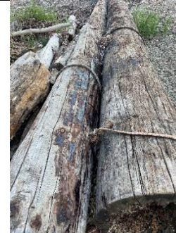
Figure 88 - Creosote logs will appear darker than natural logs, often with dark patches where the creosote is seeping out of the interior. RC4S Imagery.
