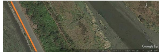
Figure 40 An example of riprap in front of a road in an estuary. Image © Landsat/Copernicus via Google Earth imagery captured 8/18/2016.
